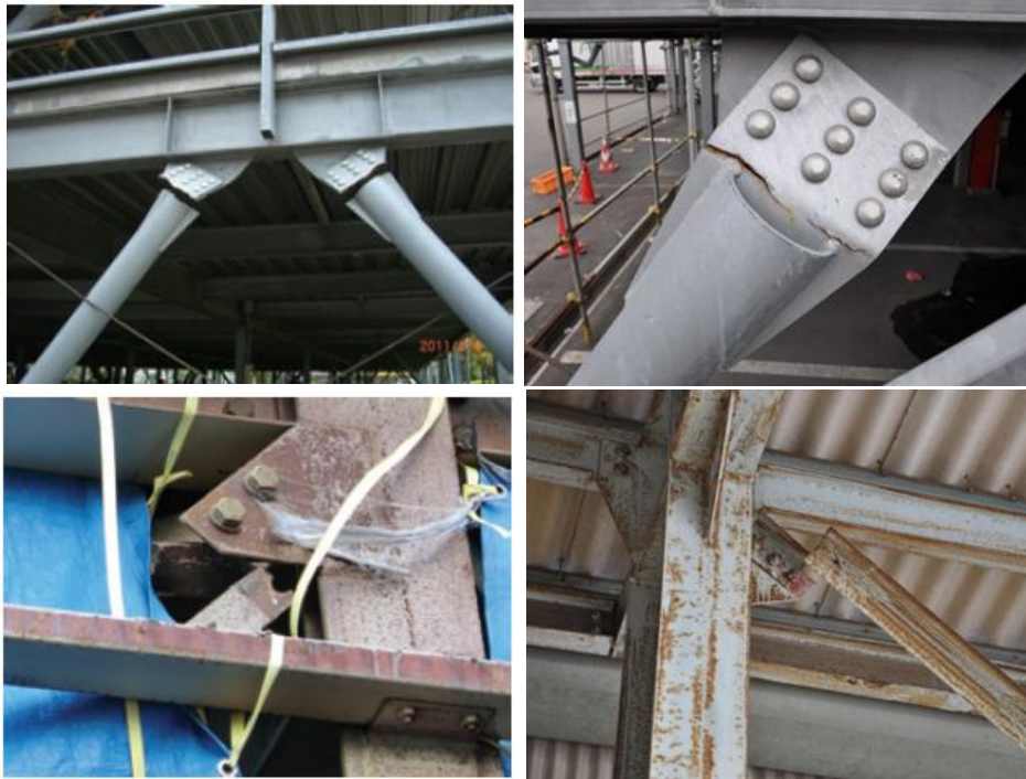
Fig. 1 – Concentration of hinge lines within the gusset plate (upper two). Brittle failure in the net section (down two).
