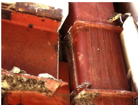
c) Damage from Kobe earthquake
